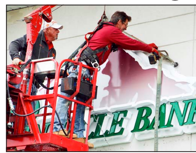
Tim Massengale and Bobby Cepeck of Masstar Signs out of Greenville, South Carolina, installed new signage and Friday at Pinnacle Bank, formerly Southern Bank & Trust of Blairsville. Photo by Shawn Jarrard
